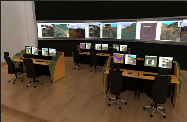
Sala de Control Principal
